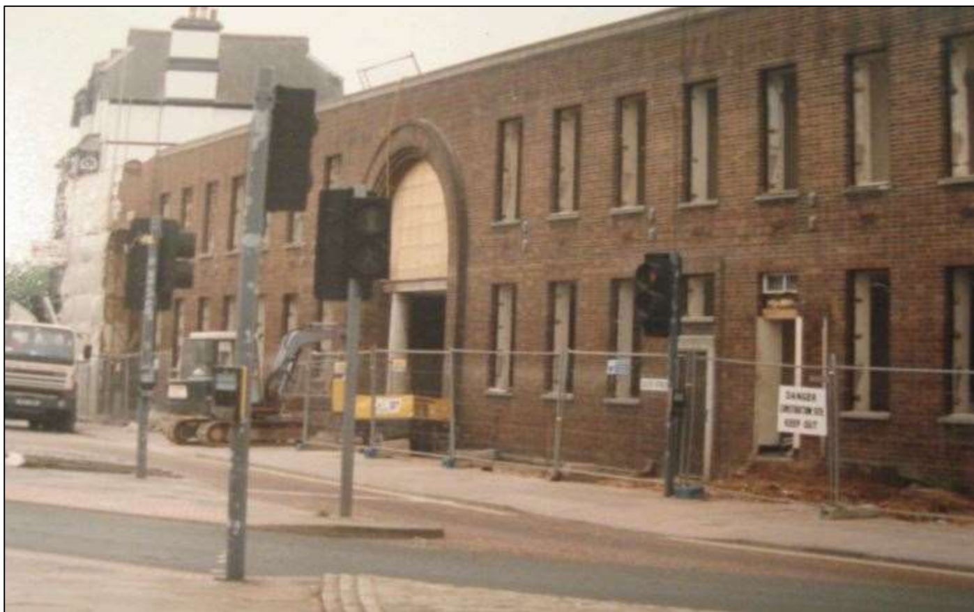
Torquay nick during the 1999 refurbishment which saw the demolition of the top floor and a significant reduction in office space. (© Paul Martin)
