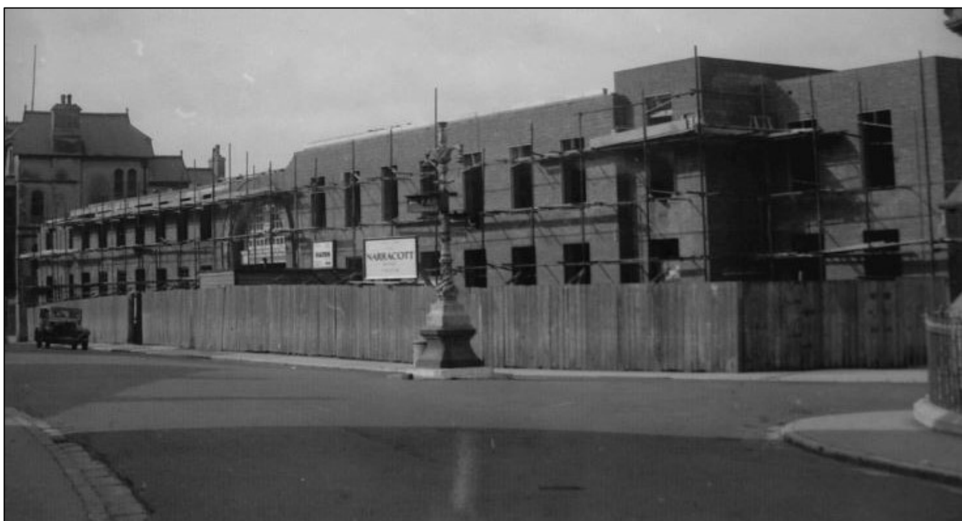
Torquay Police Station under construction. Building was paused during the Second World War. (Image courtesy of Paul Martin)
